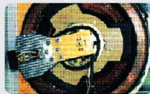
Voltage Regulating Tranformer
